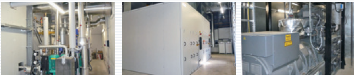
The new cogeneration unit
